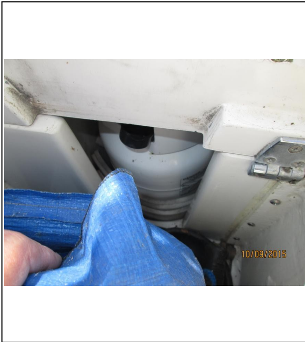
Propane locker exposed to center locker.
