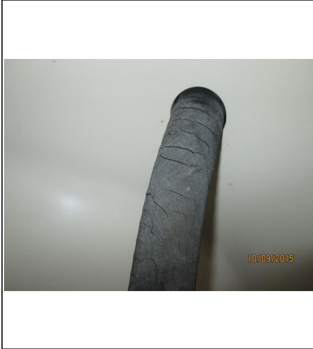
Cracked raw water hose for head.
